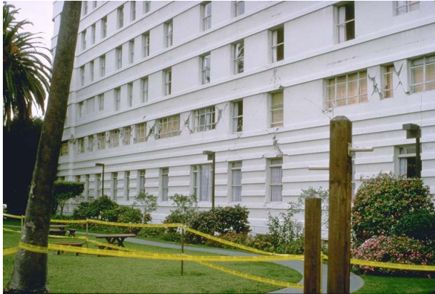
Fig. 1: St. John’s Hospital damaged in the 1994 Northridge earthquake.
